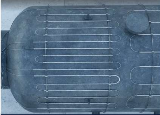
— μSTMapS Top Side Installation on Reactor
